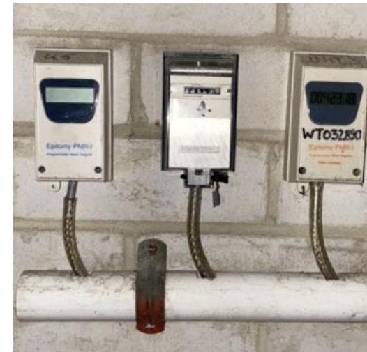
Legacy hot water meters with digital display
