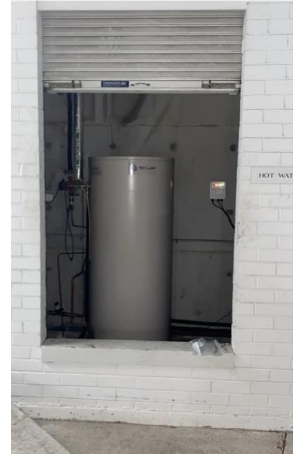
Tank for heat pump
