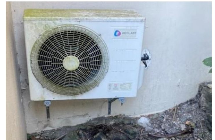
Solar & Heat Pump Projects
