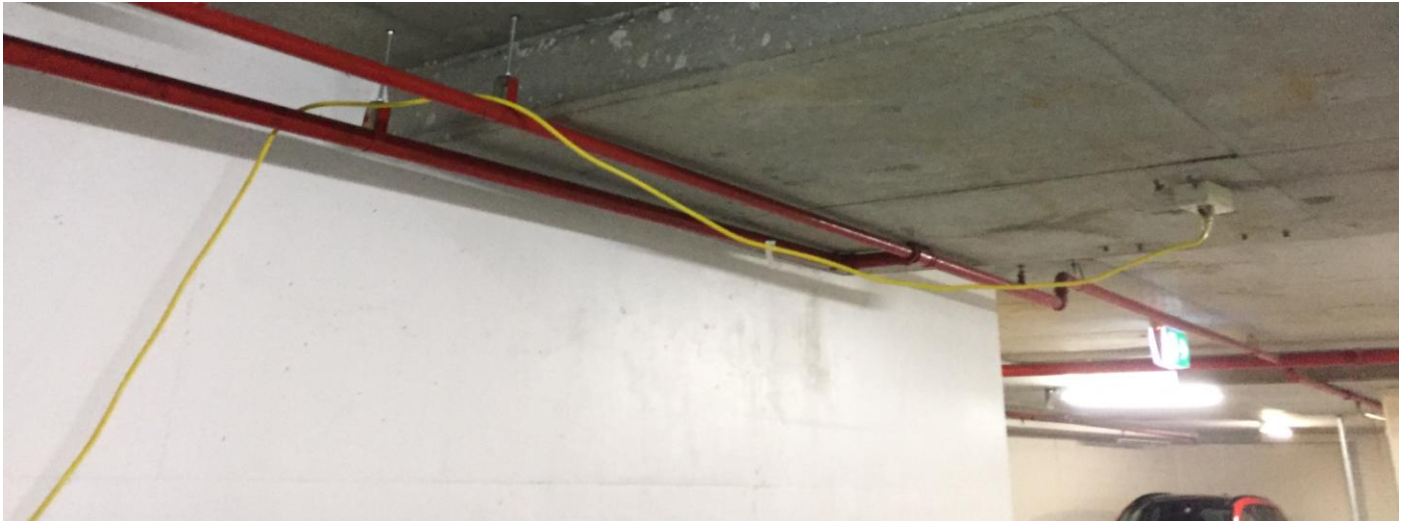
Figure 43: De-facto electric vehicle charging work arounds
