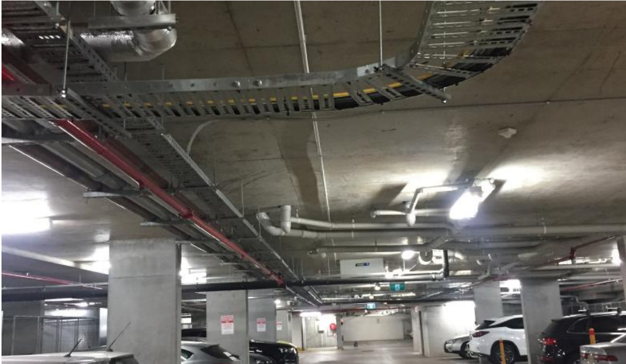
Figure 39: Sample: Cable trays installed along car park roofing
