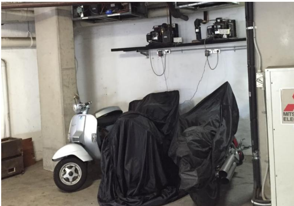
Figure 8: Electric mopeds being charged in a strata building
