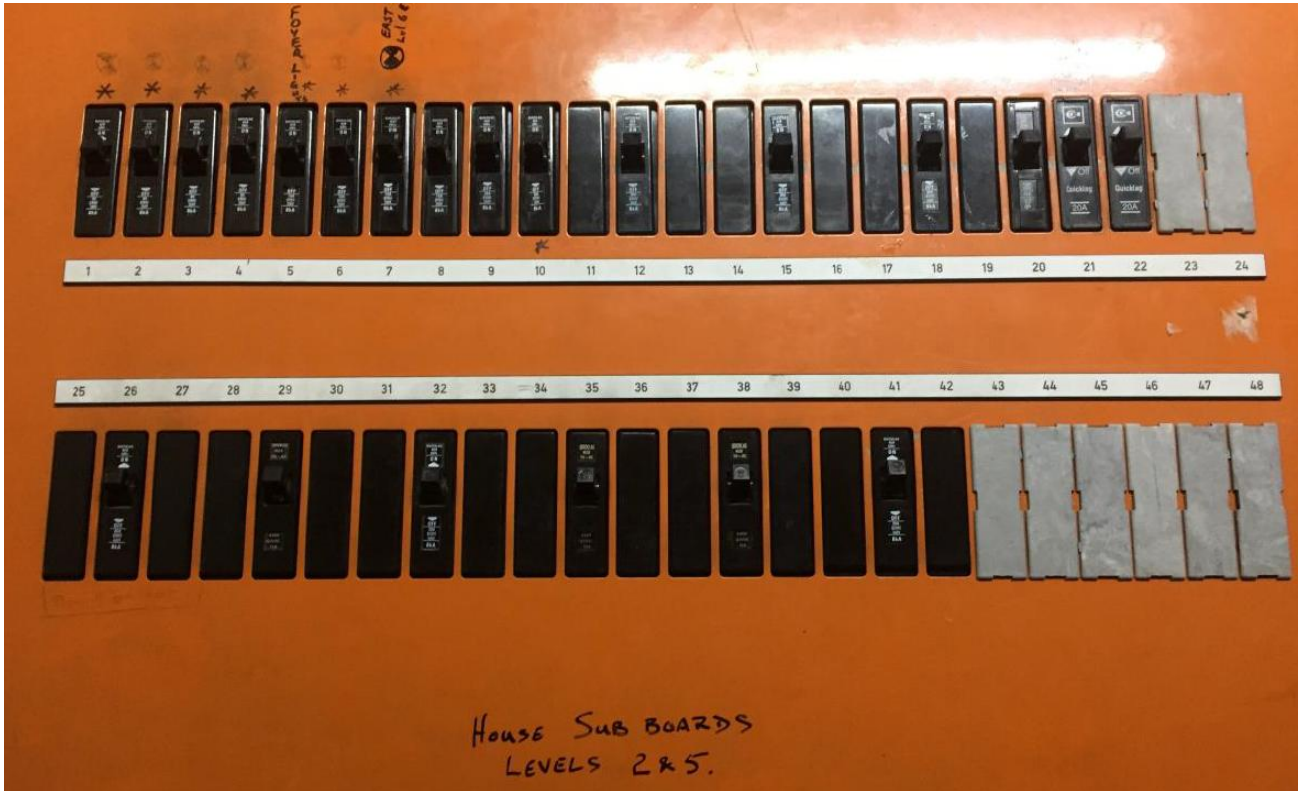
Figure 28: Sample: Distribution board
