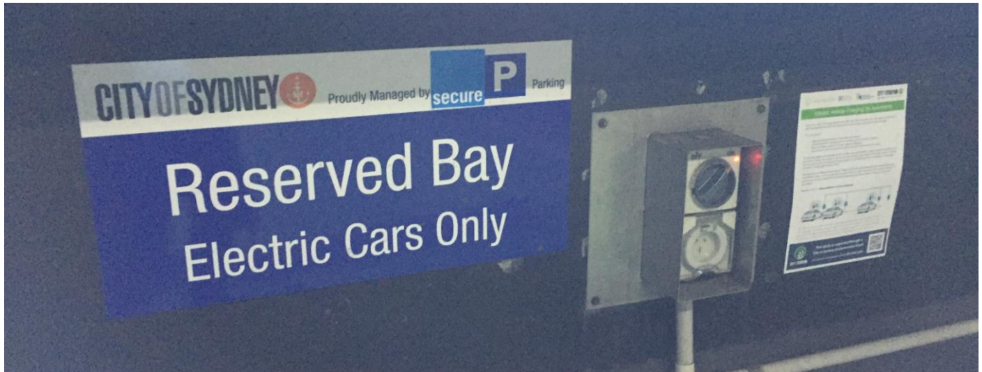
Figure 53: Poster located next to public charging facilities
