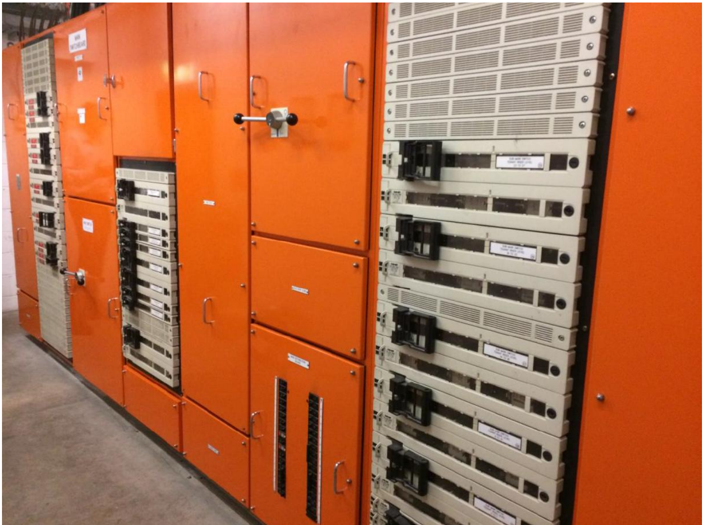
Figure 26: Sample – Main switch room
