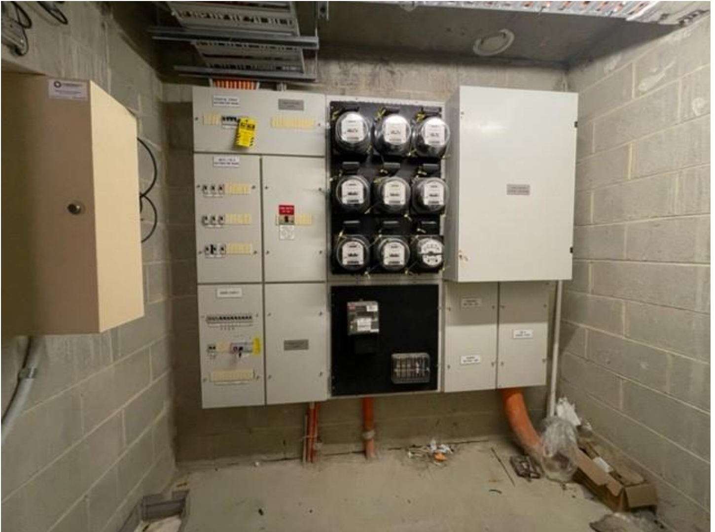
Figure 1 – Main Switch Board (MSB) located within the switch room.
